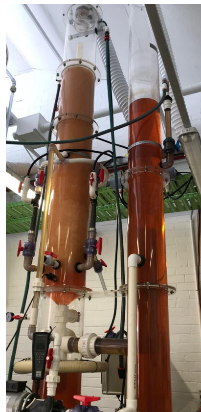
AMD Water in Treatment
