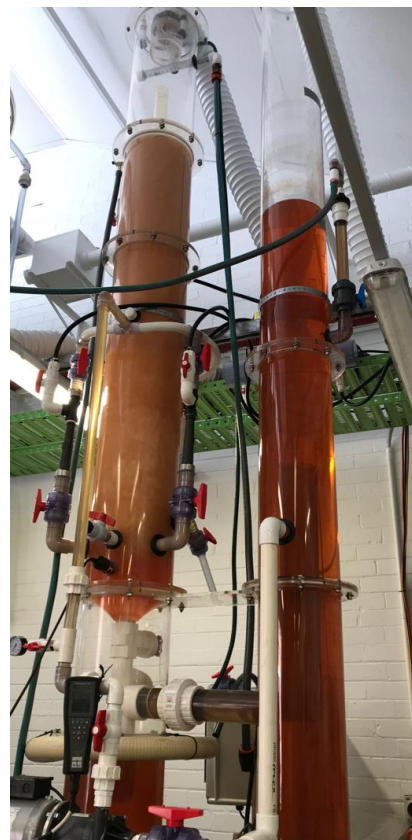
AMD Water in Treatment
